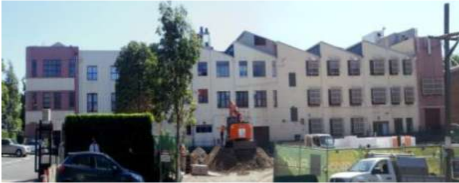
SERVICES BUILDING (G12) GFA 6,529 m 2 1920s heritage factory building, double brick construction, 3 level offices, with contemporary roof modifications for plant room spaces
