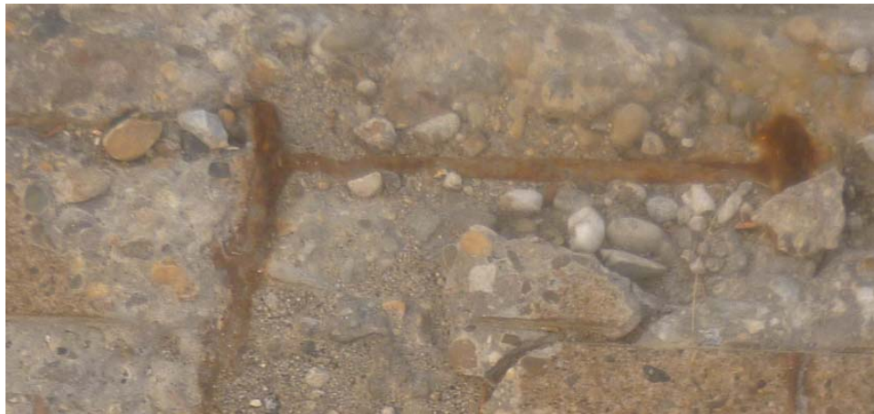
Figure 6. Example photo of corrosion of reinforcing steel.
