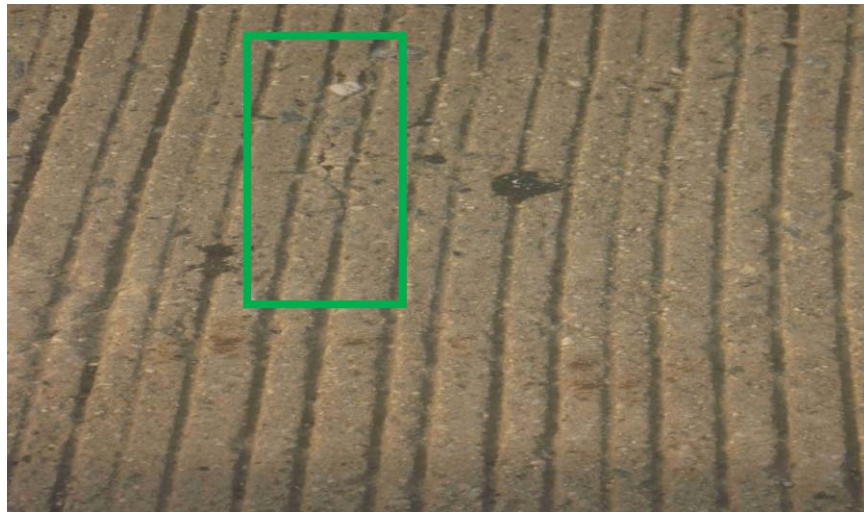
Figure 10. Example of shrinkage and creep cracks.
