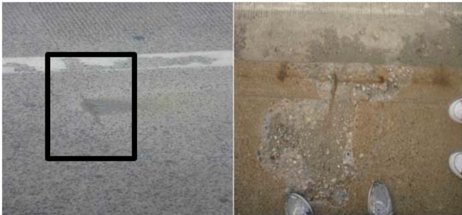
Figure 13. Examples of corrosion cracks.
