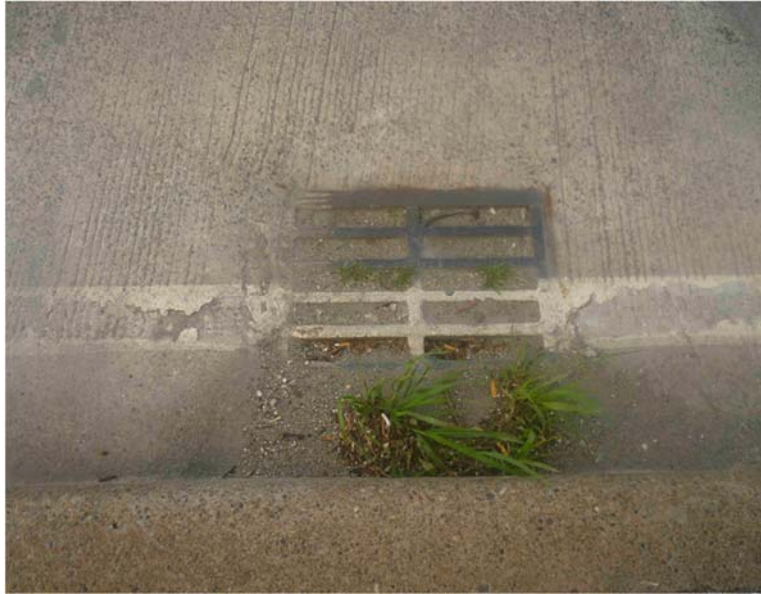
Figure 16. Example of blocked scupper.
