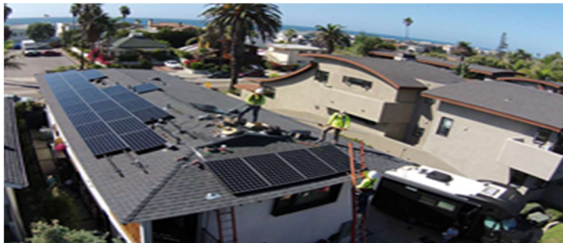
Figure 16 Solar installation industry
