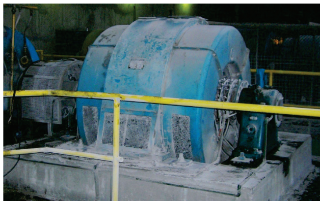
Figure 8 The 1.6 MW power electromotor in the cement plant Kakanj
