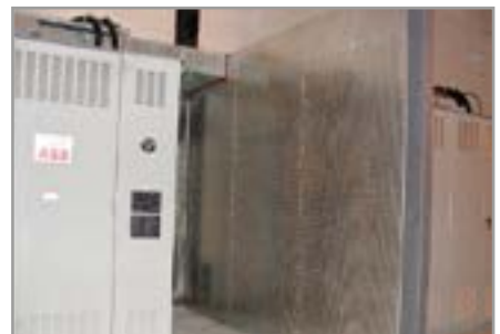
Figure 8. Critical equipment separation wall
