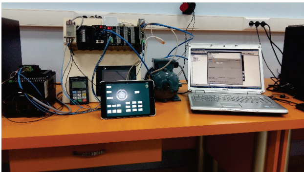
Figure 16 General view of the asynchronous motor control system
