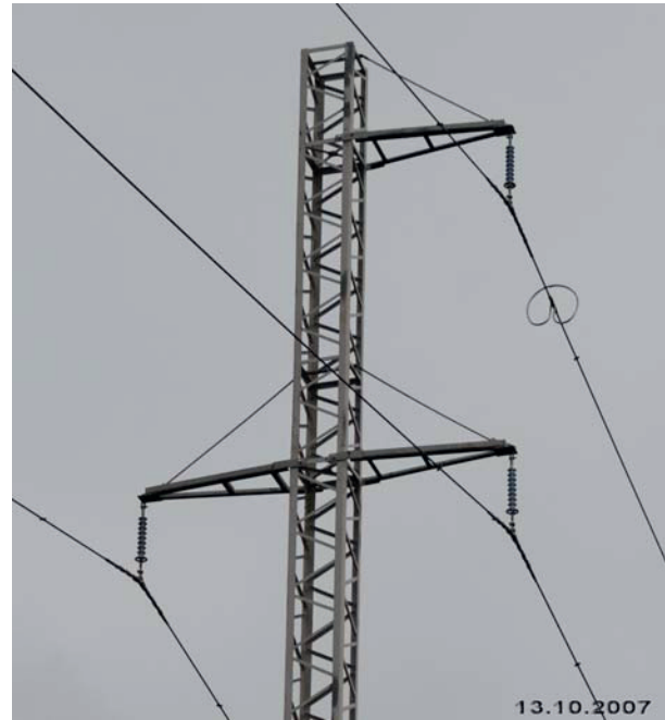
Fig. 8. 35 kV covered-conductor overhead line with Long Flashover Arresters of Antenna type.
