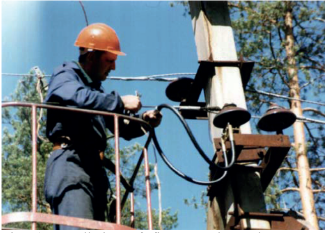
Fig. 4. Installation of first experimental arresters (LFA-Ls) in St. Petersburg utility (Russia) in 1999.
