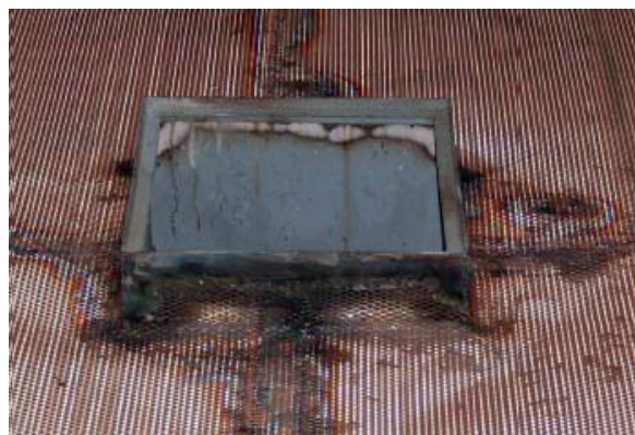
Figure 4. Cable connection box
