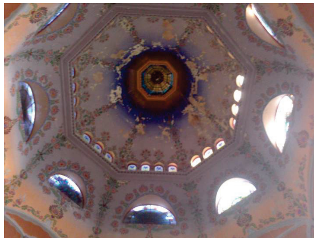
Figure 1 Damage on the vaults because of condensation
