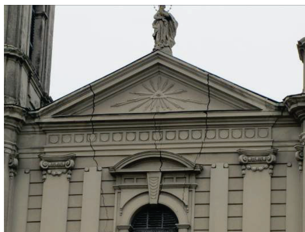
Figure 2 Large cracks on the facade of religious building
