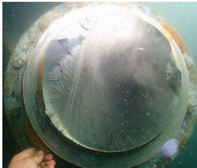
Figure 7 Uniaxial Fatigue Failure Crack Shape [15]
