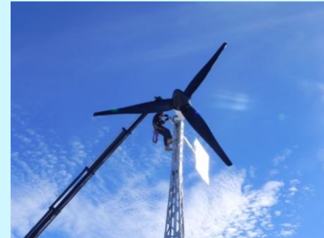
Maintenance engineer up a 12m turbine at South Africa's SANAE IV base. Credit http://www.doctorross.co.za
