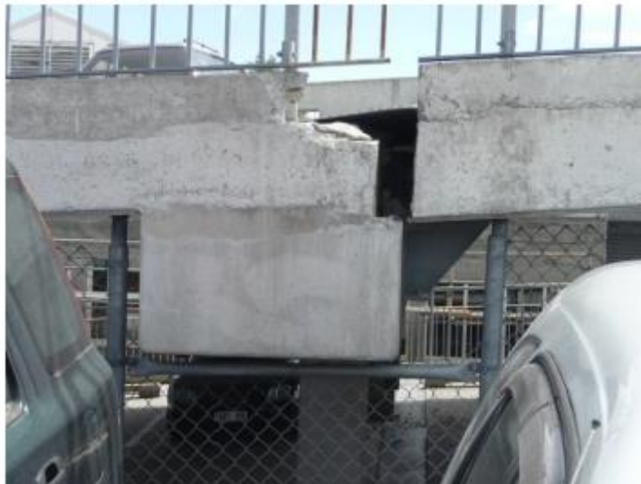
Figure 3.4. Displacement of Expansion Joint (Clifton et al. 2011)
