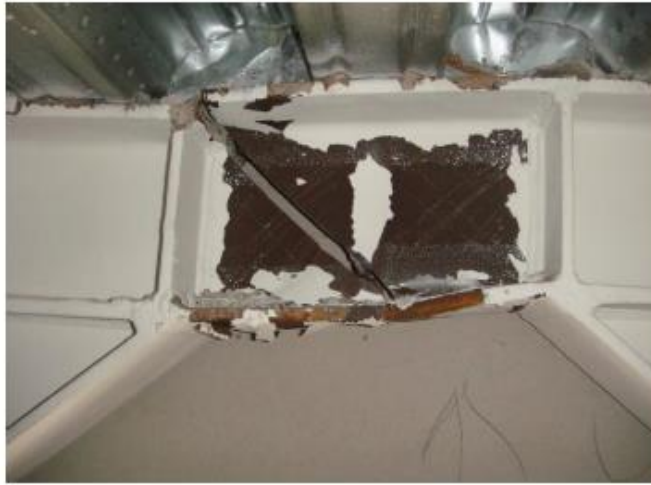
Figure 3.1. Fractured EBF Link (Clifton et al. 2011)
