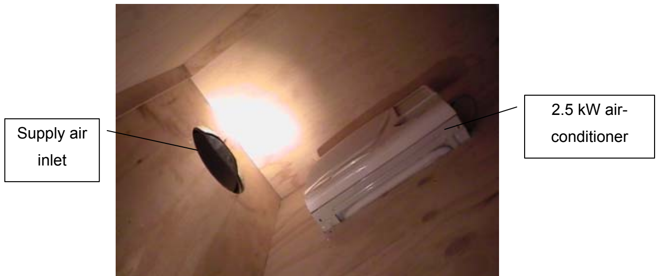
Figure 22 - Air-conditioning unit and plenum supply point
