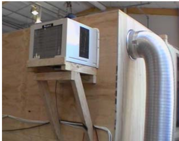
Figure 23 - Air-conditioning unit and plenum supply from outside the compartment
