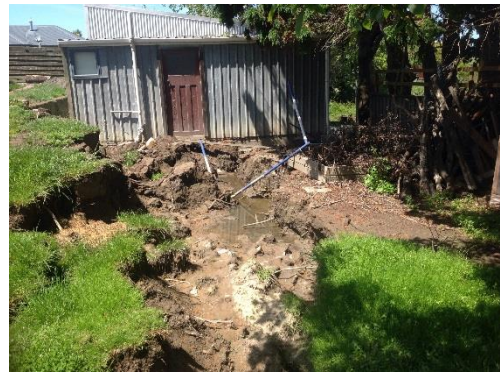
Figure 30: A garage/shed at a house on Beach Road displaced ~1 m towards Lyell Creek, and moved downwards ~ 1 m ( -42.3860^\circ , 173.6783^\circ , taken facing S).
