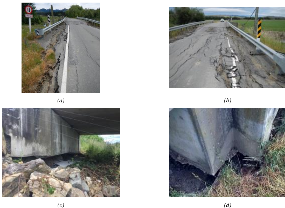
Figure 53: Settlement and cracking in approaches to Mt Paul Bridge ( -42.64^{\circ} , 172.99^{\circ} ): (a) SW corner looking N (d) NW corner looking S. (c) Settlement and spreading of fill on north (stream) side of southern abutment (looking W) exposing severely damaged piles; (d) Settlement and soil gapping on eastern side of north abutment facing N.
