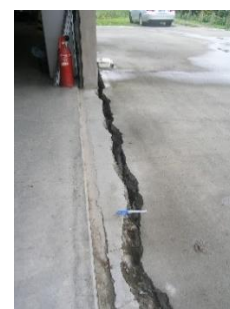
Figure 25: Separation of concrete slab from clubhouse ( -41.4768^{\circ} , 173.9855^{\circ} , taken facing N).
