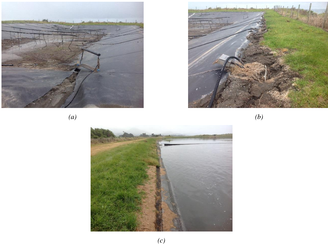
Figure 44: (a) KK-OPS looking from the SW corner. Note: Geoliner in the foreground has ripped ( -42.3668^{\circ} , 173.6865^{\circ} , taken facing E). (b) Rotation of the aeration-line control posts on the south side of KK-OPS ( -42.3669^{\circ} , 173.6867^{\circ} , taken facing E). (c) West edge of KK-OPN. Note concrete panel has displaced into pond ( -42.3660^{\circ} , 173.6868^{\circ} , taken facing N).
