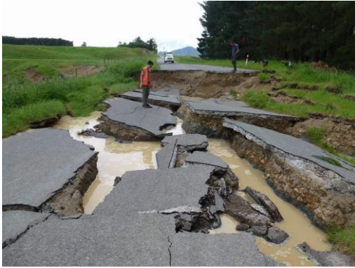
Figure 47: Damage to Leslie Hills road caused by fault rupture (Approx. coord: -42.631°, 172.990°, taken facing W).
