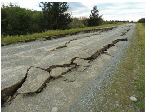
Figure 15: Lateral spreading induced cracking along top of northern stopbank ( -41.4387^{\circ} , 174.0214^{\circ} , taken facing E).
