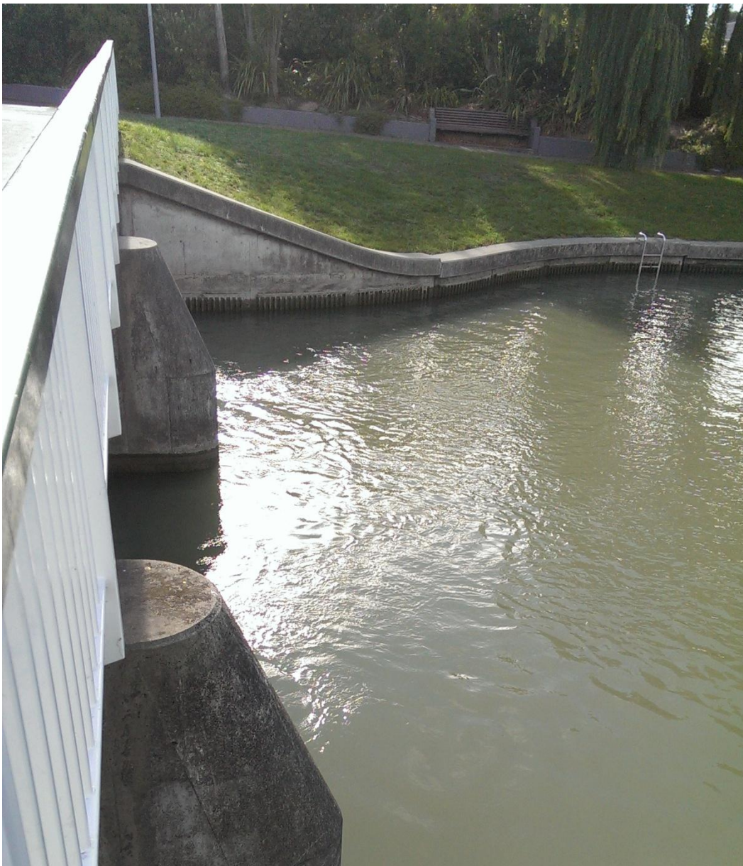
Figure 7. Observed leakage through the tidal barrage at the Woolston Cut on an outgoing tide (April 2016).
