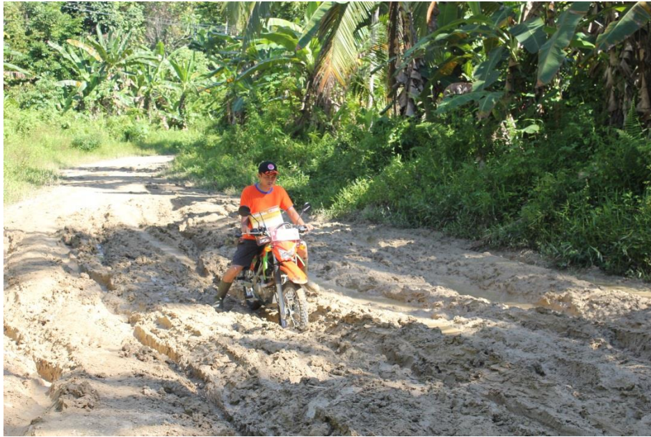
Figure 5. 2 One of many muddy points in the road from Tuapejat to Bosua (Sipora Island) Source: Personal documentation taken during the field study
