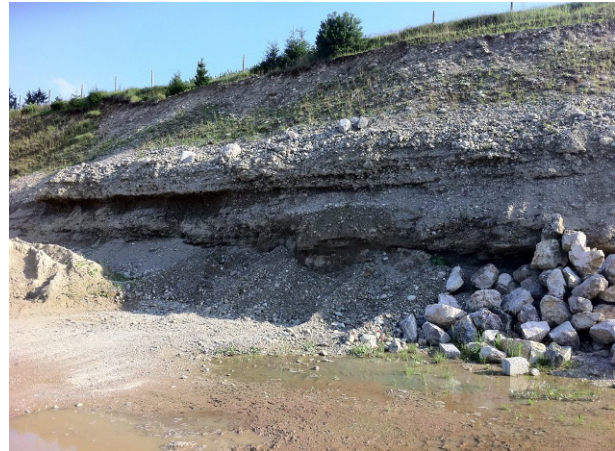
Figure 5. Gravel pit in the area of investigation showing intercalated cemented Nagelfluh layers. The thickness of the layers is between the order of centimeters and a few meters, and the cementation varies between weak and very strong, like concrete.
