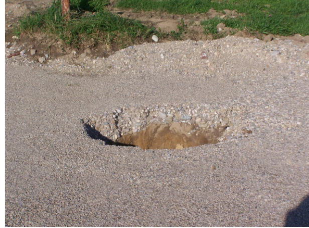
Figure 3. A 1 m-diameter Thunderhole freshly collapsed during construction works.
