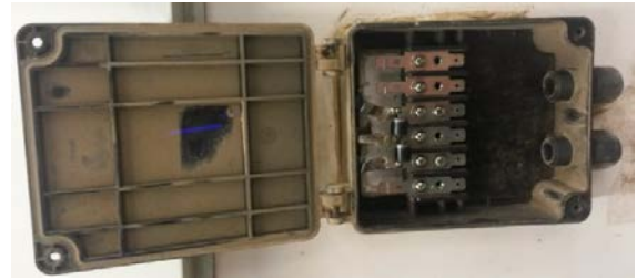
Fig. 6: Open junction box, belonging to one of the exposed modules, claiming IP65 protection against dust and water ingress.
