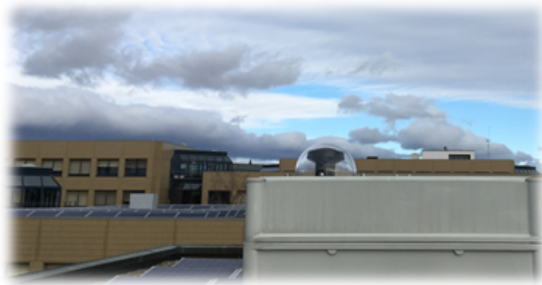
Figure 4.2 – Basler all-sky camera installed on the rooftop PV plant at the EPFL DESL laboratory.
