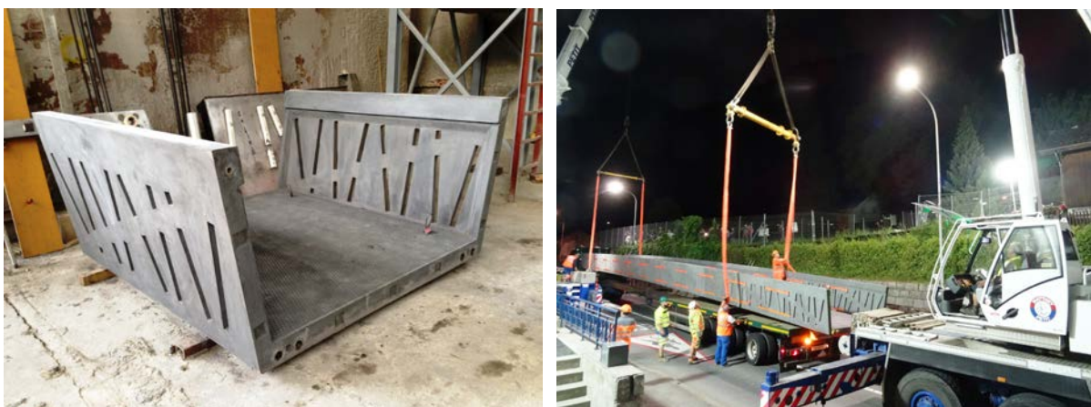
Figure 14. Precast UHPFRC element in the plant (left); lifting of the assembled girder by two cranes in the night of May 25, 2018.
