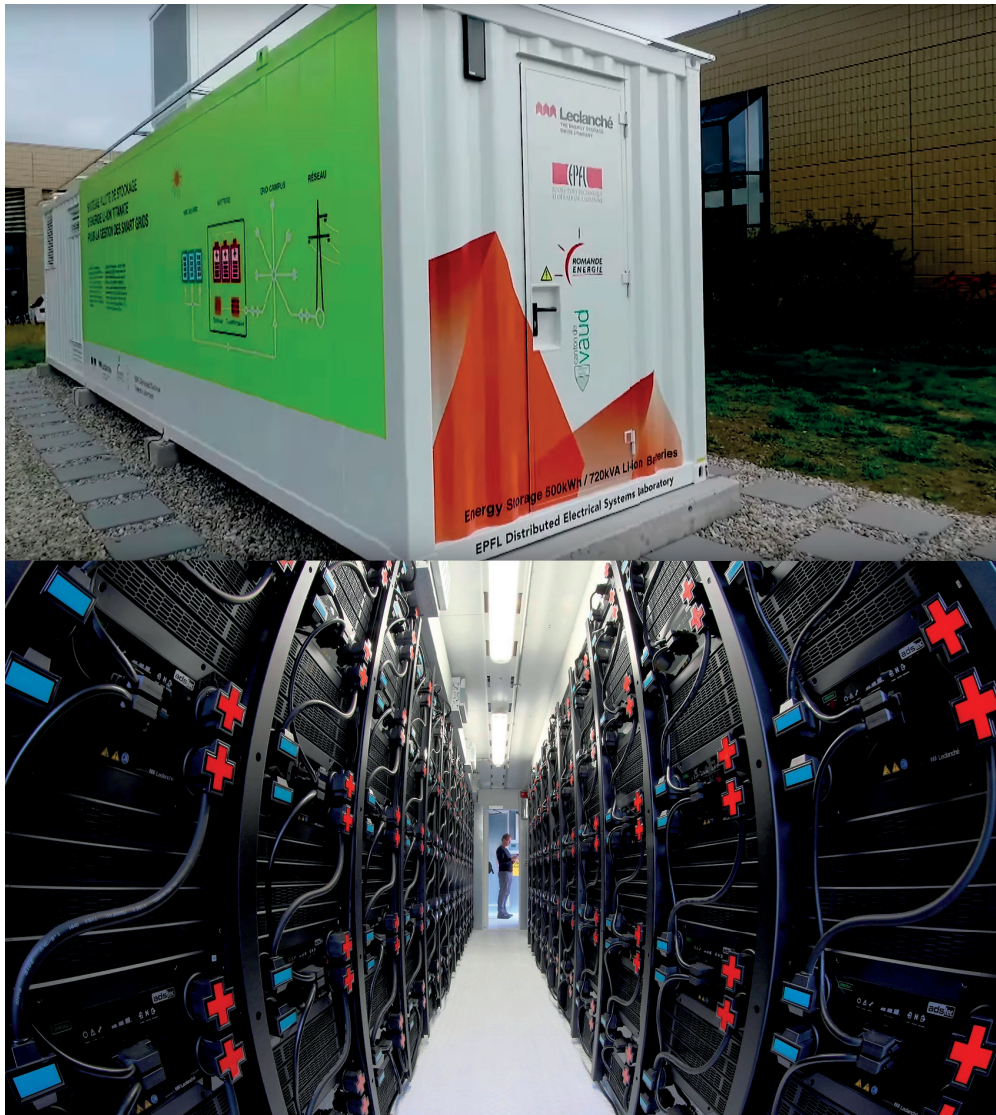
Figure 1.3 – An outside (top picture) and inside view (bottom picture) of the 720 kVA/500 kWh Lithium Titanate-based BESS installed at EPFL (picture of Alain Herzog, EPFL).
