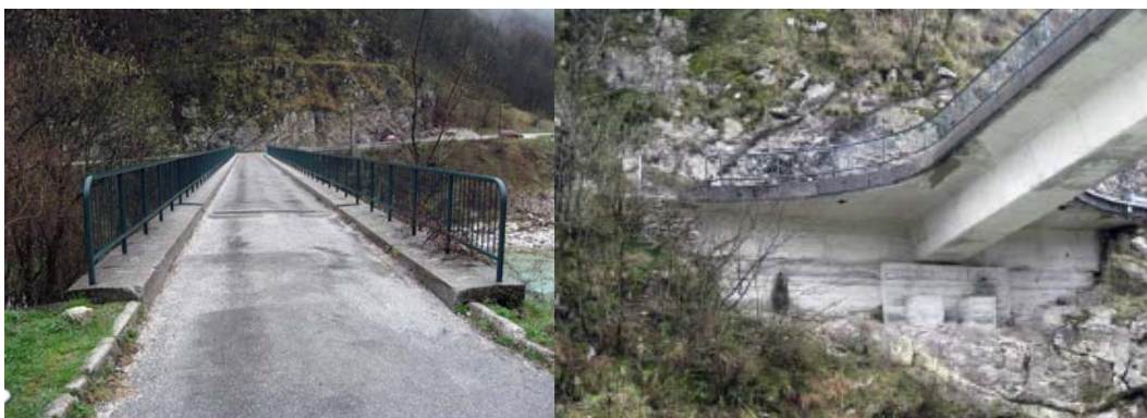
Figure 4: Overview of the bridge, deck, and lower face close to abutment, prior to rehabilitation.
