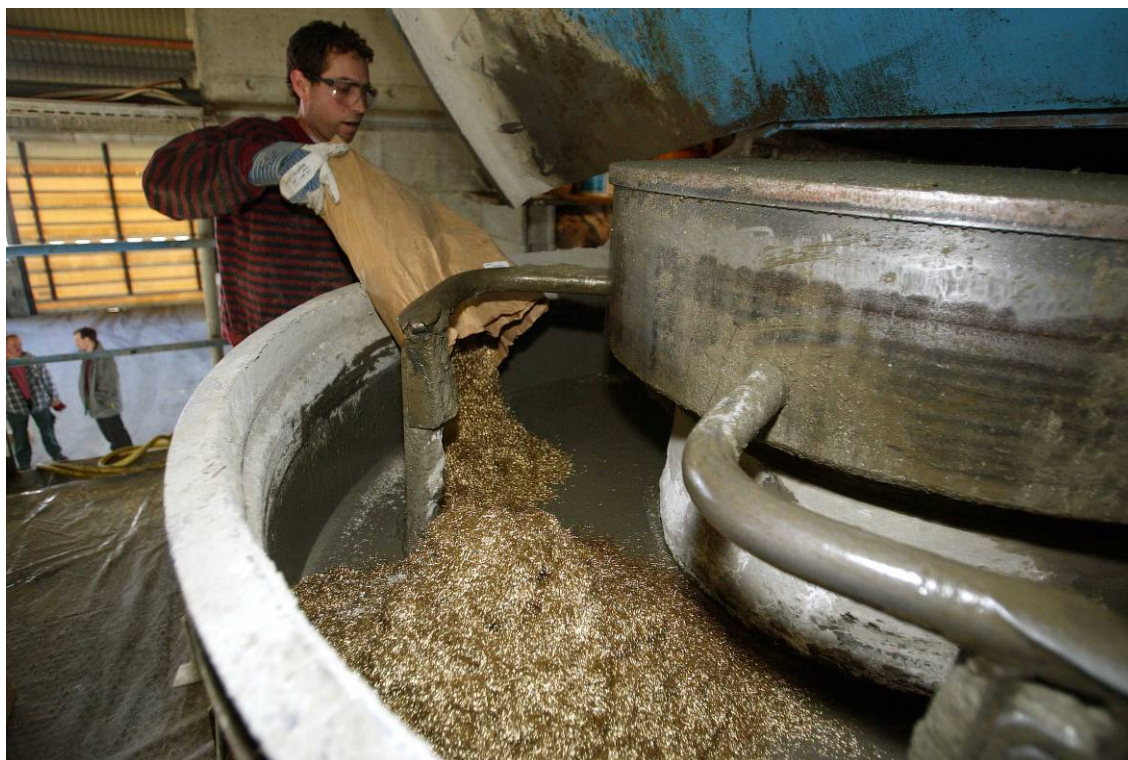
Figure 13: Fabrication of the UHPFRC (adding of the steel fibres) in a common mixer of the prefabrication plant (Photo A. Herzog).
