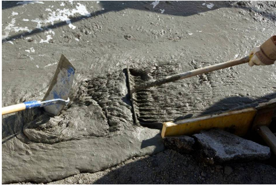
Figure 18: The thixotropic, selfcompacting UHPFRC, is handled using simple tools (Photo A. Herzog).
