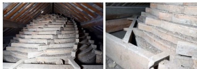
Figure 16. The space between the roof and the caisson, built in the 1920s in Ninghai. Ref. ZJ-04A © Jingxian Ye
