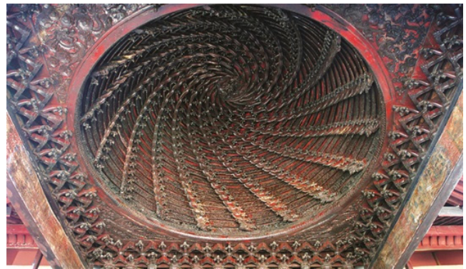
Figure 9. Spiral type: opera stage of Chenghuang Temple, built in 1935. Height: 2.1 m; Diameter: 4.1 m. Ref. ZJ-02 © Peiliang Xu
