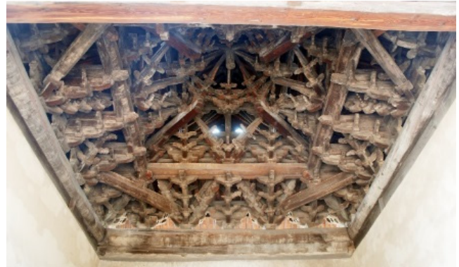
Figure 4. Caisson in Dongyang Temple, built in 1345. Width: 8.04 m. Depth: 7.90 m. Height: 4.43 m. Ref. SX-02 © Jingxian Ye
