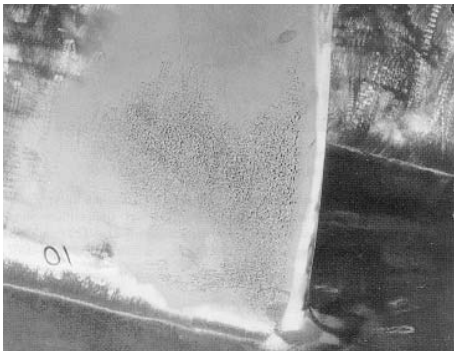
Fig. 28 "Frosted" area at the wall of the runner blade trailing edge due to outlet traveling bubble cavitation, shaded area C of Fig. 25.
