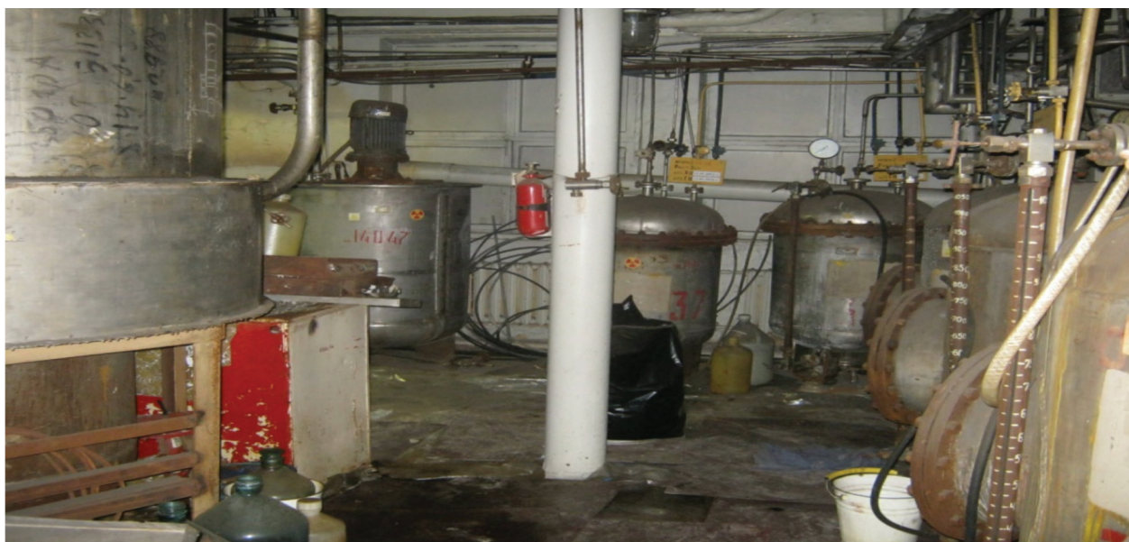
Figure 1. Radiochemical facility equipment.
