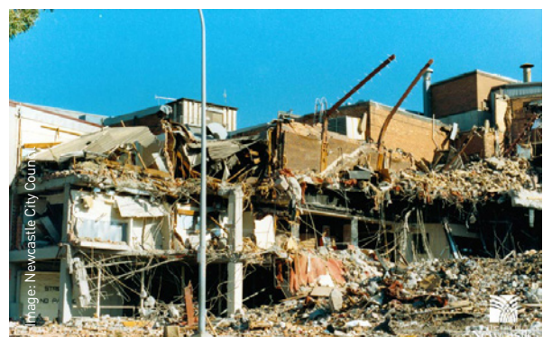
Demolition of Newcastle Workers Club, the scene of the greatest damage to any building in Newcastle where nine people died and many others were injured.
