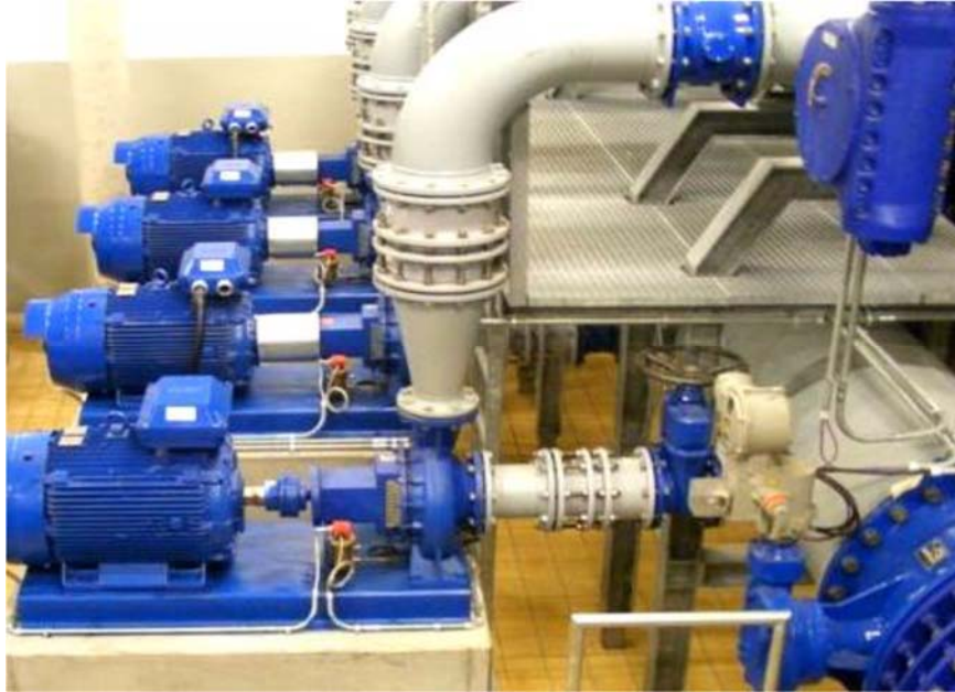
Figure 4-47 Four of eight parallel PATs in service at the water utility authority (Zweckverband Landeswasserversorgung, Stuttgart, Germany) [16]
