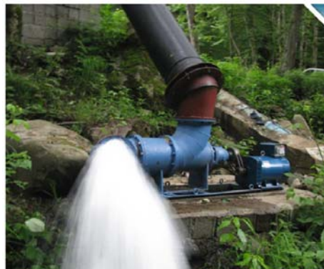
Figure 3-5 An axial PAT based micro hydropower station, installed in the North of Iran [2]
