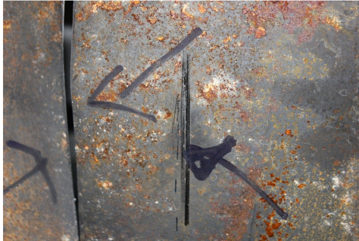
Figure 4.3: Bearing Contact Damage (shown to the right of the fracture)
