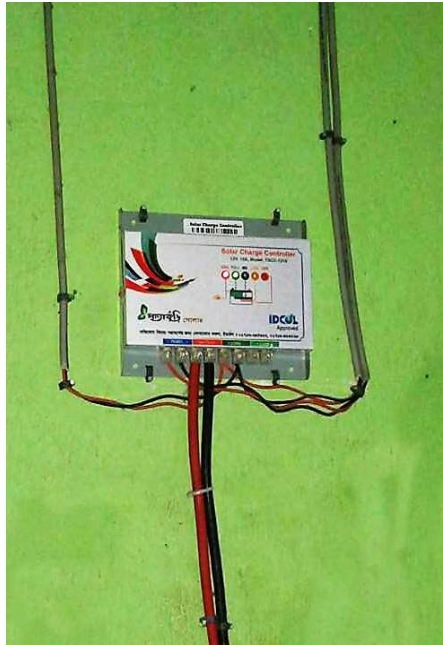
Figure 2- 5: Pico-Solar Charge Controller Setup in the House Wall
