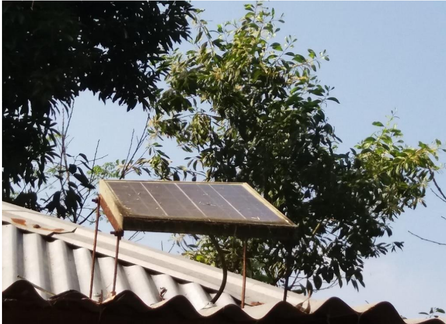
Figure 2- 4: Pico-Solar Panel Set Up on the House Roof
