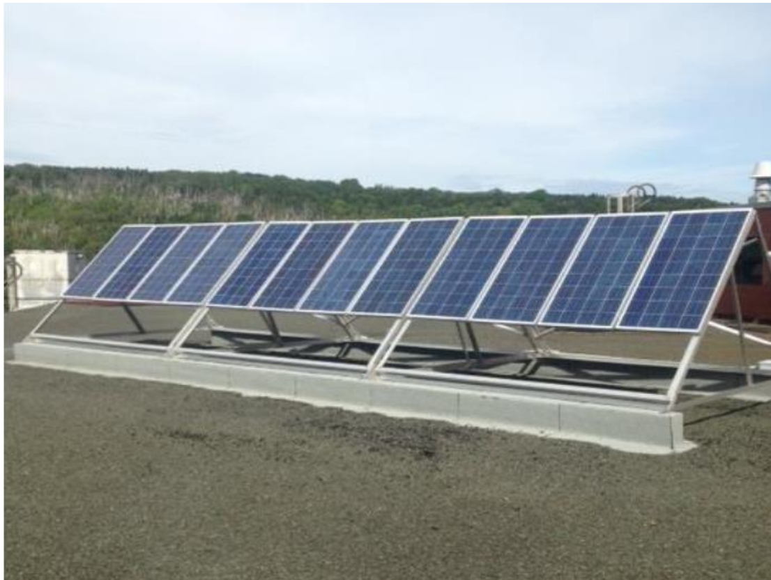
Figure 3- 9: Solar Panel Installed in Engineering Building
