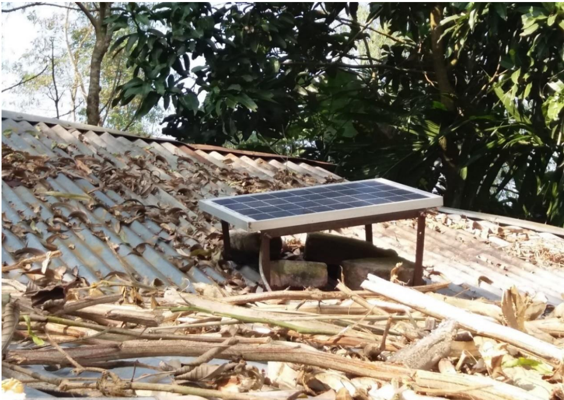
Figure 2- 2: A Rooftop pico-solar panel of a rural house in Sreemangal, Sylhet, Bangladesh.
