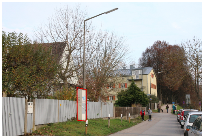
Figure 12.: A circuit breaker panel located next to street is an example of a non-building included in the sample. The picture was taken by the author and a red frame was added in order to avoid misconceptions using GIMP (cf. The GIMP Team, 1997-2013).
