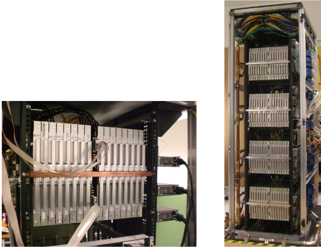
Figure 5.1: The photograph on the left shows the QPACE test setup at the IBM laboratory in Böblingen, Germany. The photograph on the right shows a fully populated and cabled rack tested in the lab.
