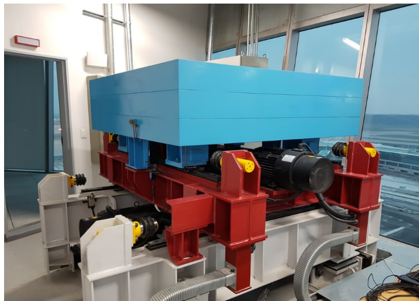
Figure 2-2 : AMD (Active Mass Damper) for Incheon International Airport Apron ATC Tower, after installation ( www.tesolution.com )
