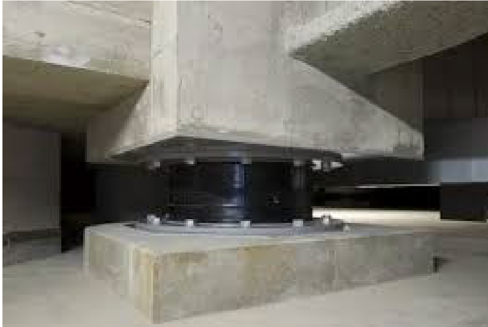
Figure 2-12 : Base isolators (LRB) installed between columns and foundation – Taiwan (Robinson Seismic www.rslir.com , June 2018)
