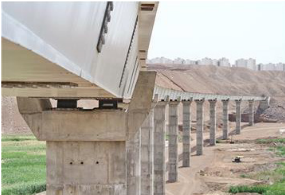
Figure 2-13 : Base isolators installed between the deck and piles of a bridge – Roudshour -Saveh –Iran (Robinson Seismic www.rslir.com , June 2018)
