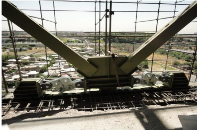
Figure 2-5 : Rotational friction damper installed in a building –Tehran-Iran (Damptech www.damptech.com, June 2018)
