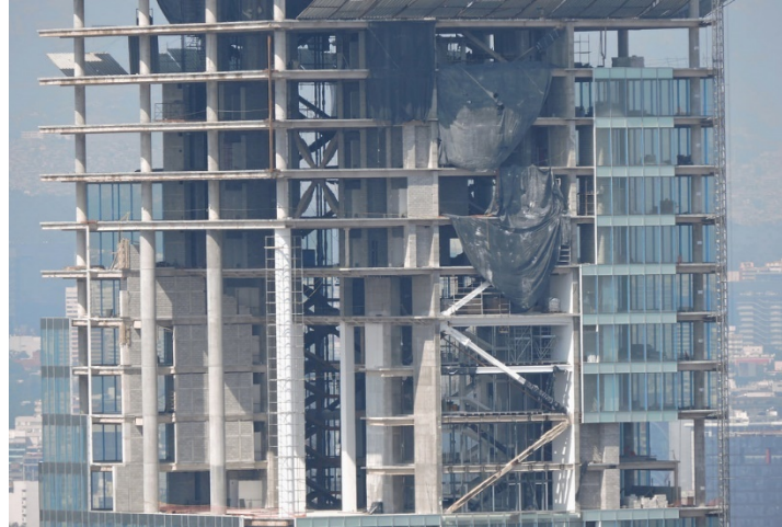
Figure 2-4 : Straight frictional dampers installed in the bracing system of a building- Torre Cuarzo- Mexico D.F-Mexico (QUAKETEK www.quaketek.com , June 2018)
