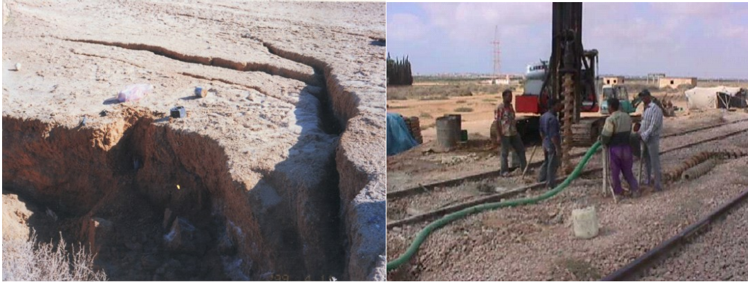
Fig. 1.2. (a) Sinkholes developed nearby the railway line; (b) Filling the voids by grouting as soil treatment (Sakr et al., 2008)
