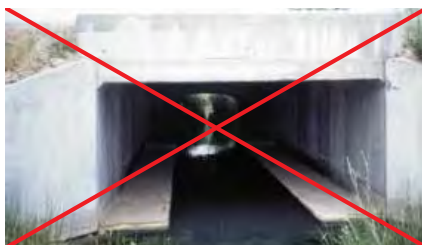
Figure 9.10. Lack of ramps connecting the dry ledges with the adjacent areas. Photo: F. Navàs.
