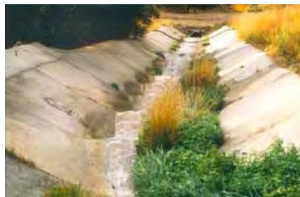
Figure 9.8. Protective culvert outlet on an embankment with sloping side walls adapted to facilitate movement by wildlife. Photo: C. Rosell.
