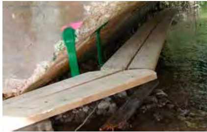
Figure 9.5. Platform that facilitates animal movement through a culvert. Photo: Development and Environment Department, Government of Castilla y León.
