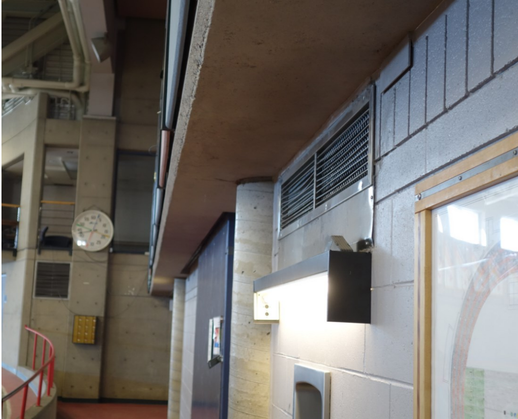
Figure 7-3. The air diffuser on the south wall of the MG building.
