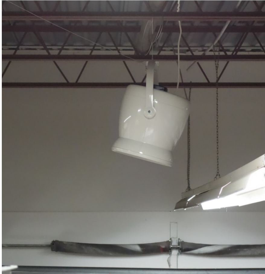
Figure 1-3. A bucket fan mounted beneath the ceiling of the QT warehouse.
