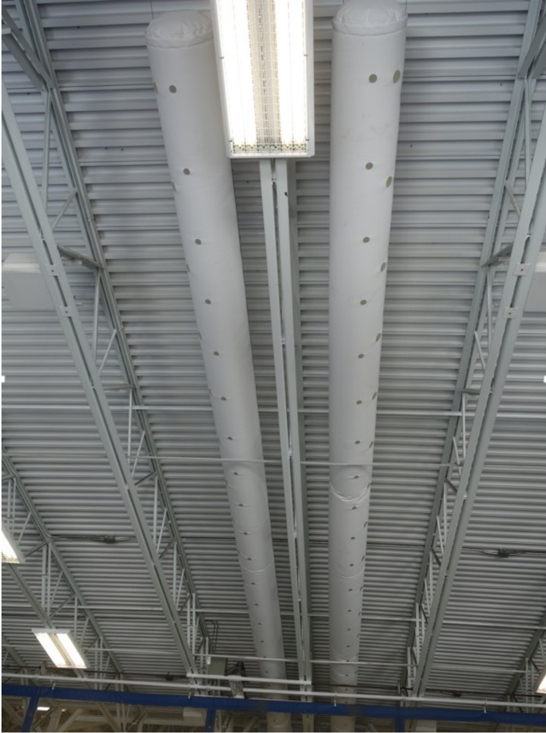
Figure 7-4. The fabric diffusers beneath the roof of MG building.
