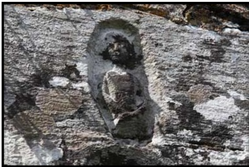
Figure 3.6 Sheela-na-gig over rounded window on the southwest side of Ballyvourney Church, County Cork; Web < http://www.megalithicireland.com/ >
