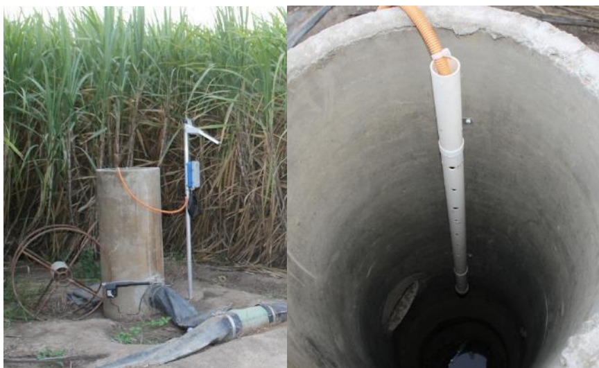
Figure 6-8 – Pressure transducer installed at Pozzebon site.
