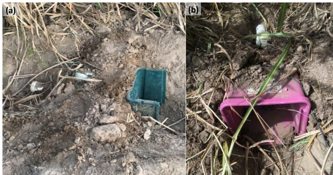
Figure 6-39 – Elster Q4000 flowmeters installed in the furrow (a) side view and (b) front view
