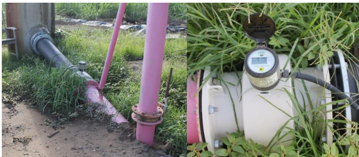
Figure 6-23 – New Siemens flowmeter at Linton pump 2.
