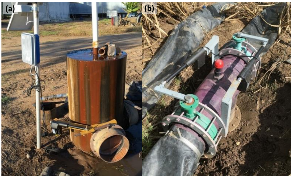
Figure 6-18 – Valves on (a) cylinder and (b) closed riser at the Linton Site.
