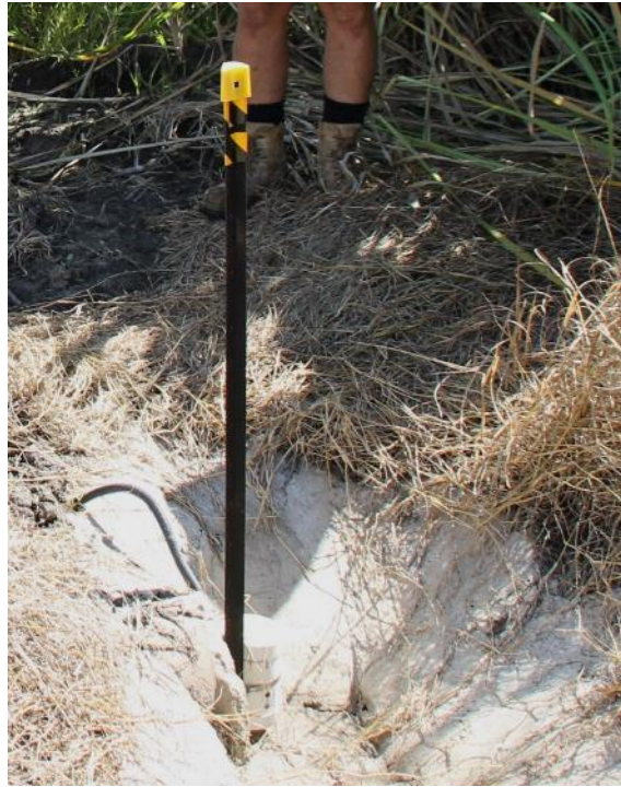
Figure 6-14 – Drain sensor installed upstream of culvert at end of blocks 3 and 4 at Pozzebon site.
