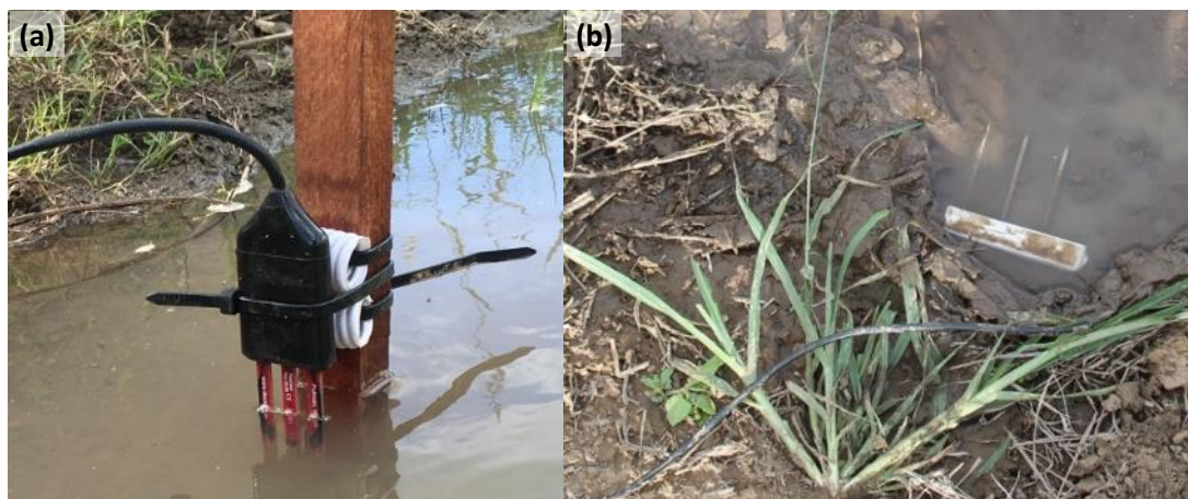
Figure 6-28 – 5TM Soil moisture probe (a) and GS3 soil moisture probe (b) installed as temporary drainage probes
