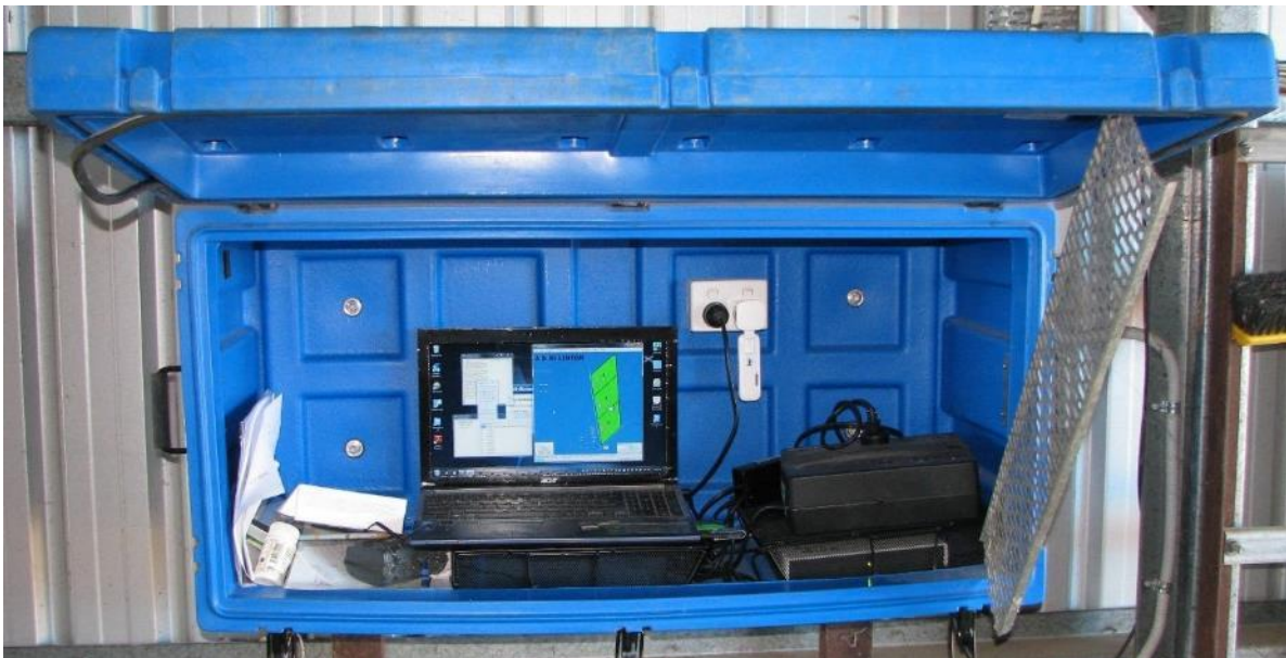
Figure 6-1 – Base station at Linton site
