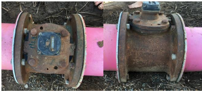
Figure 6-22 – Original flowmeter at Linton pump 2
