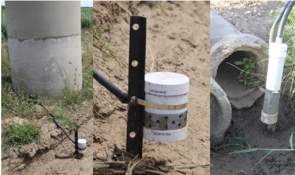
Figure 6-31 – Install site for drainage probe for blocks 5 to 8, close-up of housing for GS3 drainage probe and install of MP406 probe for blocks 1 to 4.
