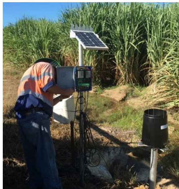
Figure 9-11 – Davis rain gauge connected to WiSA radio at end of blocks 1&2.
