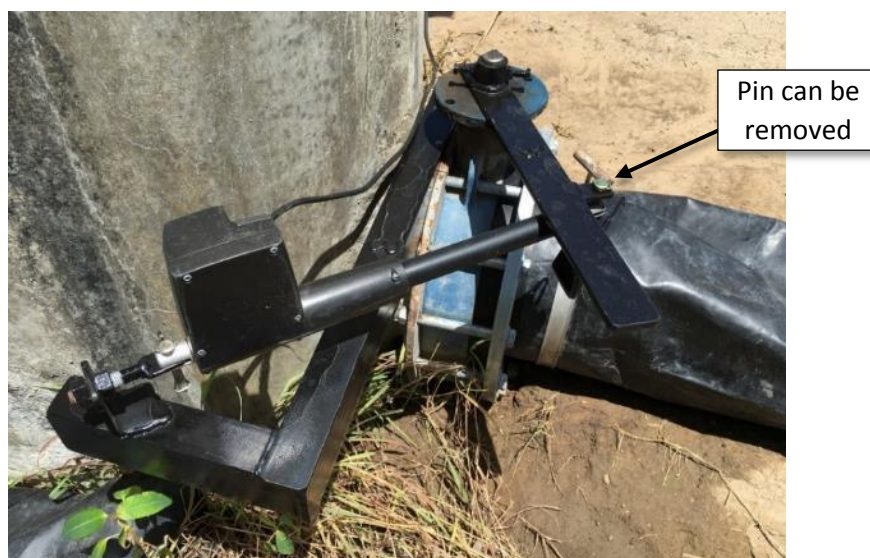
Figure 6-34 – Close up of valve and actuator at Jordan site.
