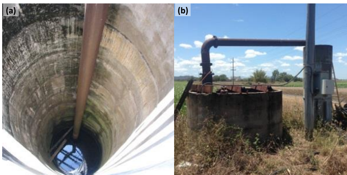
Figure 5-1 – Example of (a) shallow bore and (b) groundwater pump pumping water into concrete cylinder
