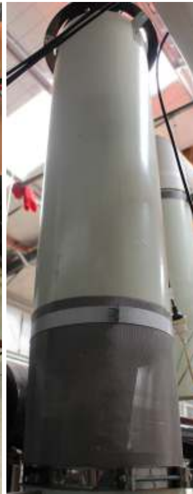
Figure 3.42: Housing for atmospheric blow-down device for fuel delivery.
