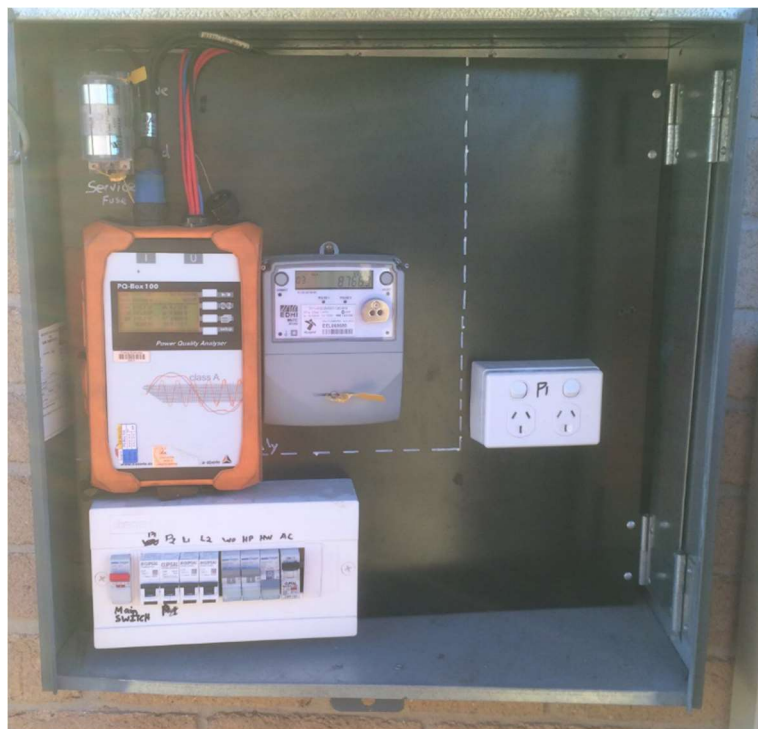
Figure 3.1 – PQ-Box 100 installed in main switch board
