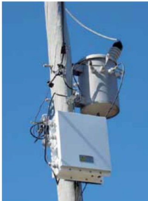
Figure 2. 1 – MicroPlanet LVR on SWER transformer by T&D
