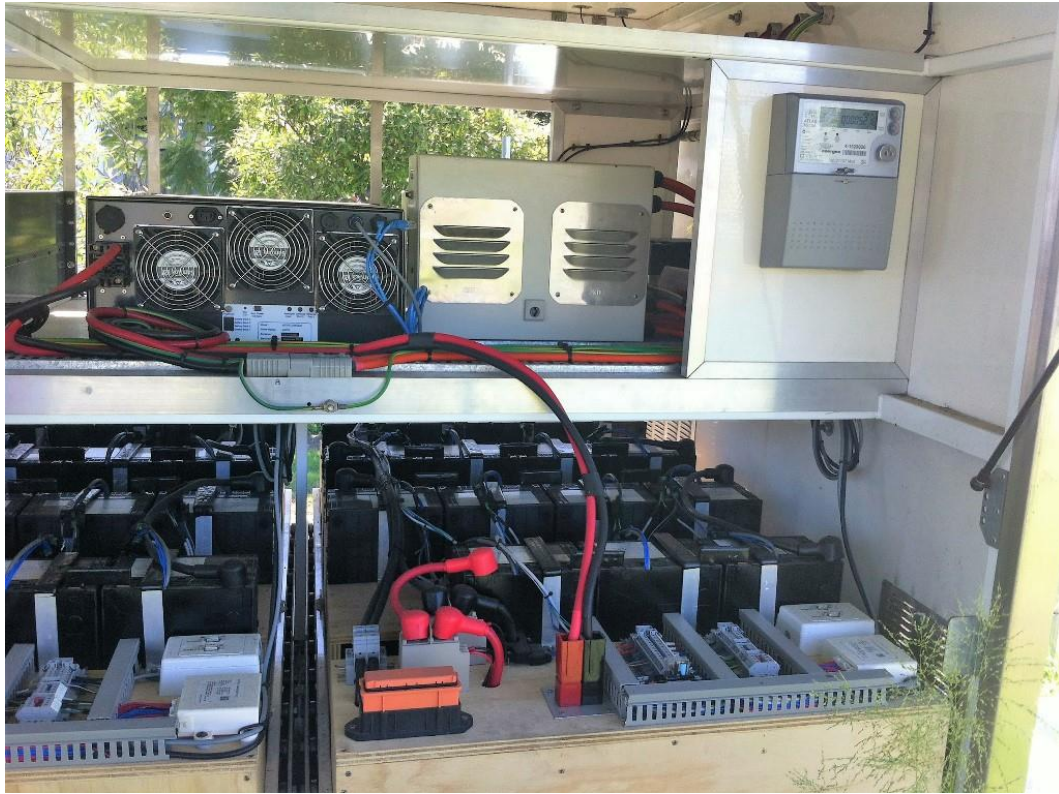
Figure 2. 6 – Batteries and Statcom unit in Energex trailer
