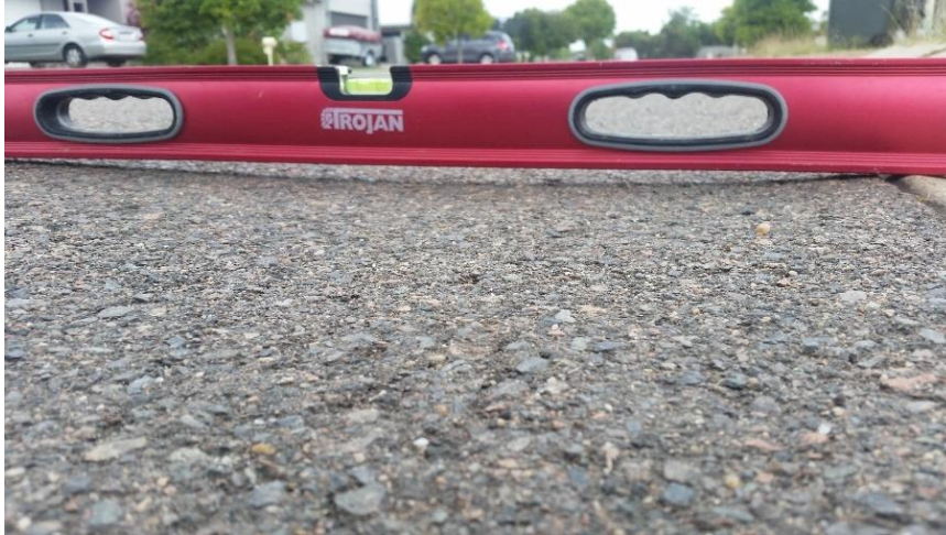
Figure 18 - Oculina Street Pavement Failure
