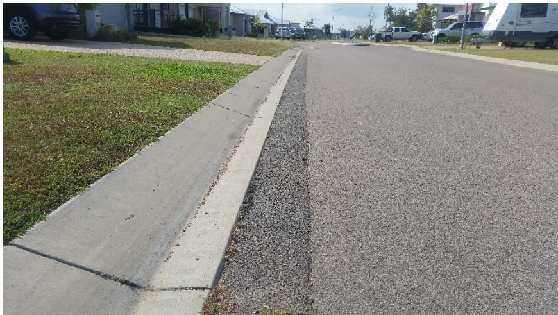
Figure 14 - Saba Street Pavement Failure
