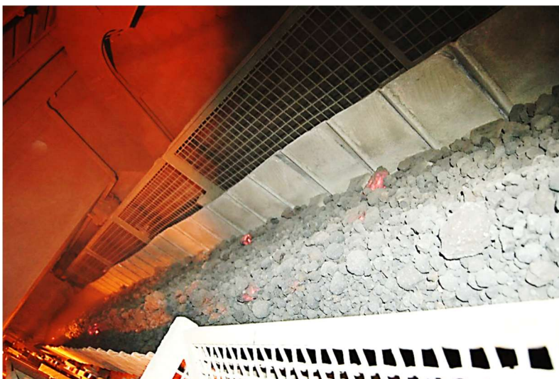
Figure 21: Clinker Sampling Station
