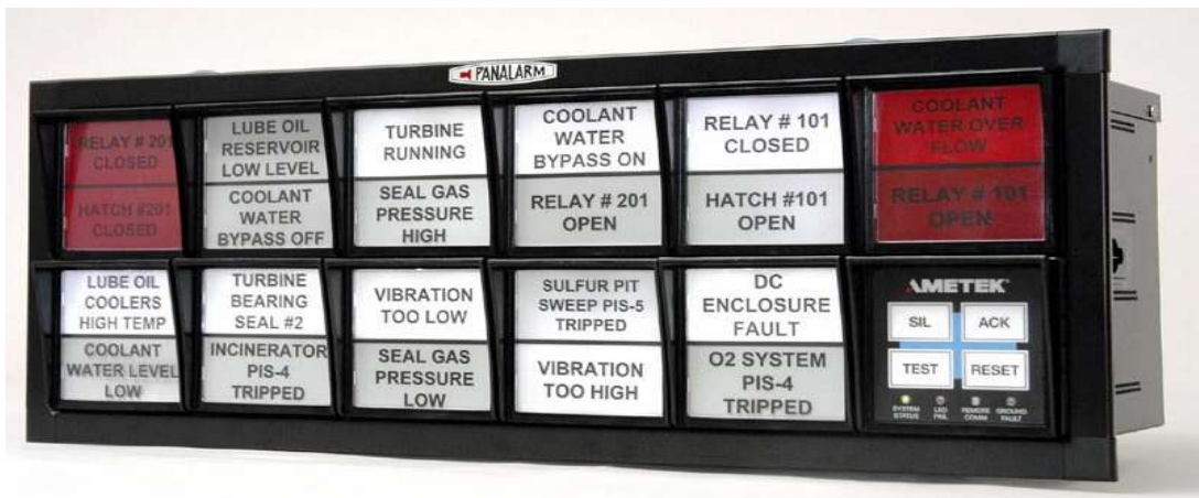
Figure 4: Example of a panel mounted annunciator (Engineered Solutions, 2012)
