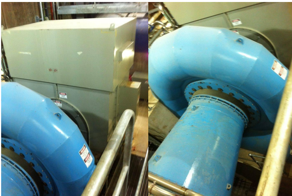
Figure 3.5; Photo's 5 & 6 Turbine generator
