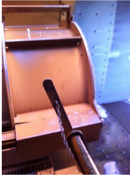
Figure 3.6; Photo 7- Dissipation Chamber
