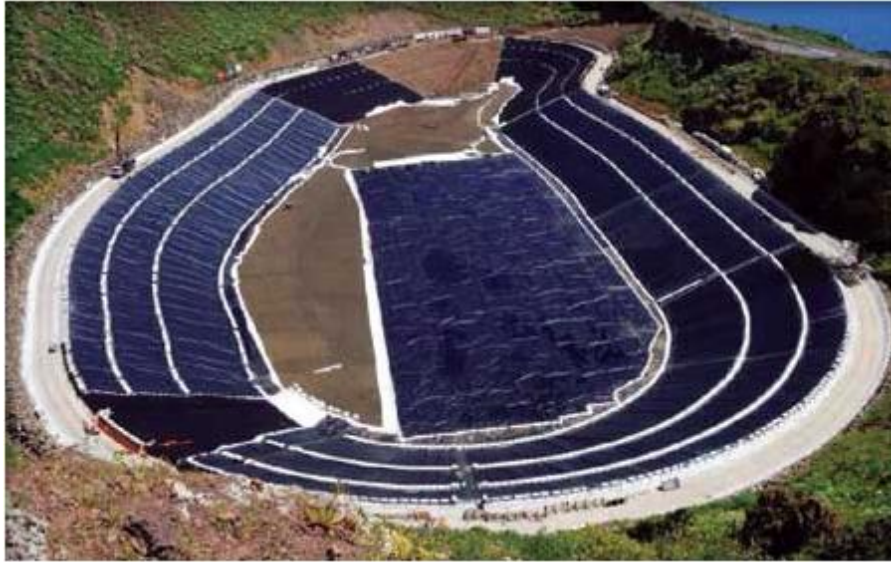
Figure 2.21: Geo-membrane for waterproofing (minimises seepage) (Hydro Review, 2012).
