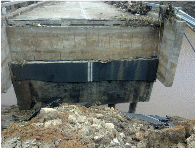
Fig 1: Damaged Kapernicks Bridge in Lockyer Valley Region in Queensland, Australia
