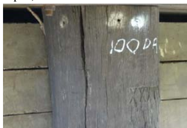
(e) Vertical splitting (overloading-top of pile)
