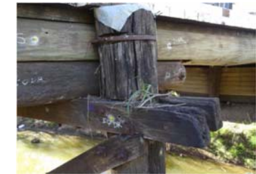
(f) Vertical splitting (changed section-top of pile)
