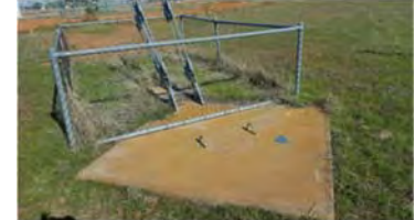
Figure 2 – Guy wire concrete anchor (Johnson 2016).
