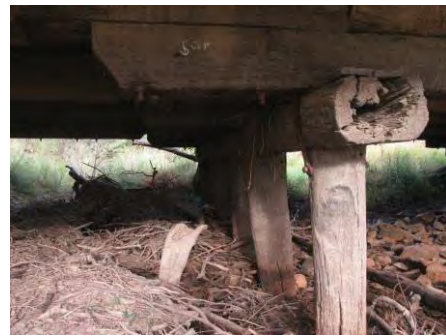
Figure 1: Tummaville Road, Leyburn bridge suffers from severe deterioration (Stark, 2016)
