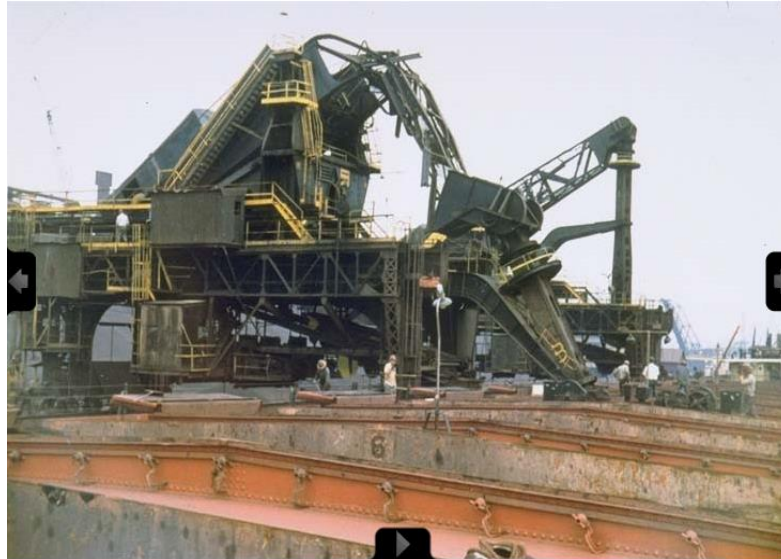
Figure 1-2: Structure failed due to fatigue (Leap Australia 2014)
