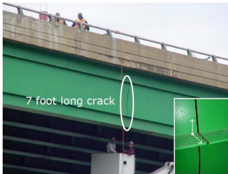
Figure 1-3: Fatigue cracking in a bridge girder from weld defects (Haghani 2012)
