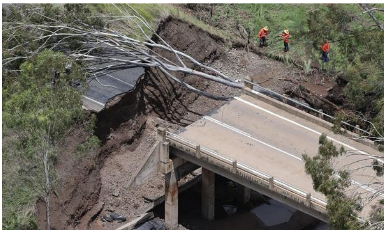
Figure 2-3: Cyclone Marcia Damaged Bridge in Gladstone Biloela Rd
