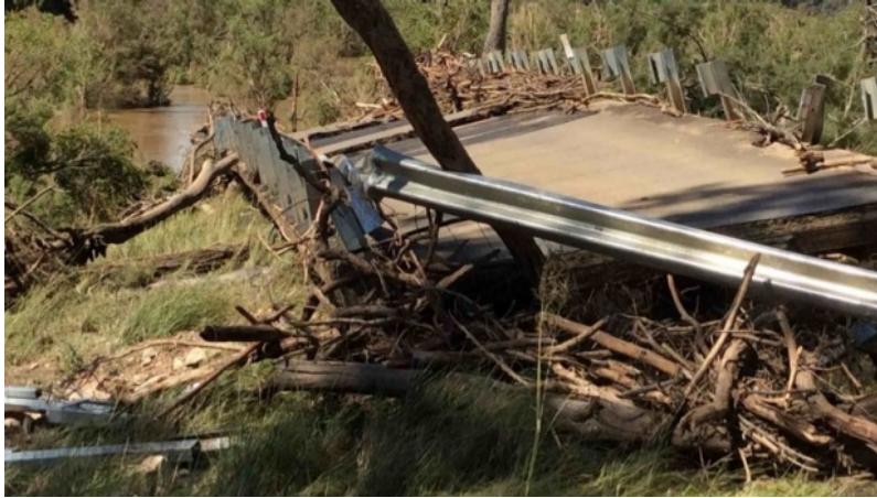
2: Cyclone Marcia Damaged Bridge in Monto
