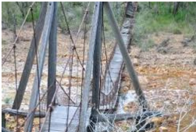
Figure 2-4: Cyclone Marcia Damaged Bridge in Mount Morgan
